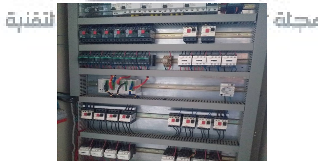
Figure -1 control panel HMS for house Number F-2
